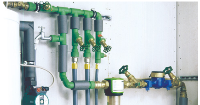
House connection station
